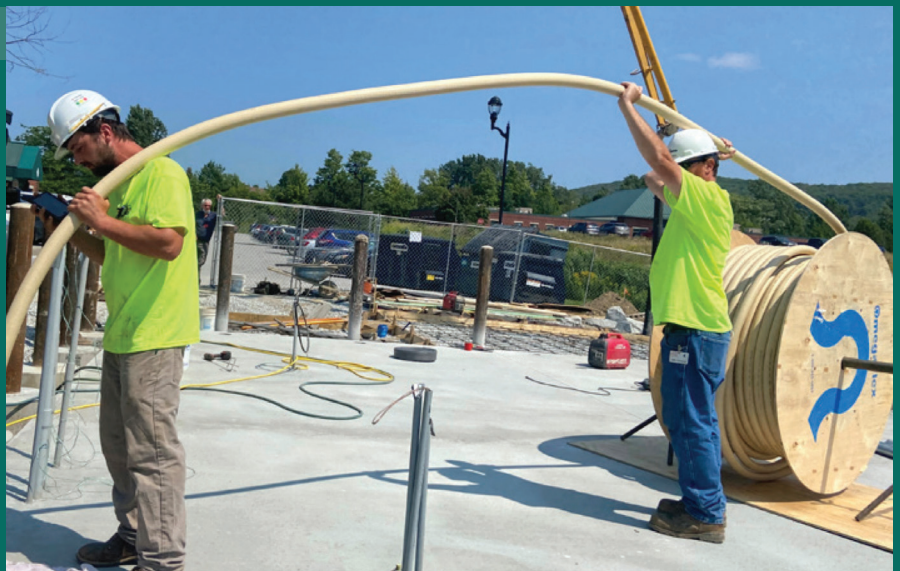
Oxygen main line for medical center.
